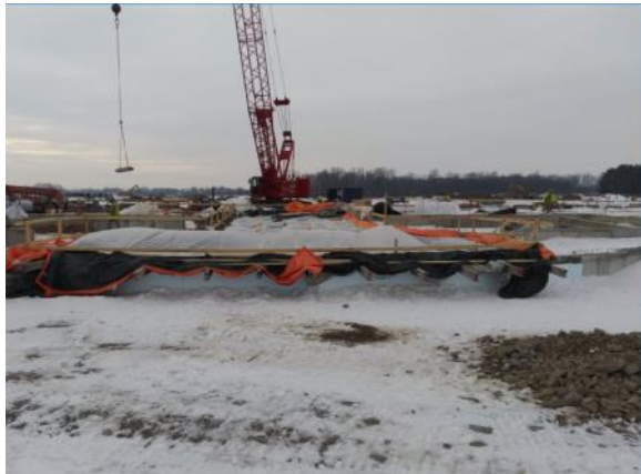
Future orchestra pit is covered with blankets to allow concrete to be poured in cold temperatures (12/13/2021)
